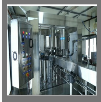
40 BPM Rinsing, Filling and Capping Plant
